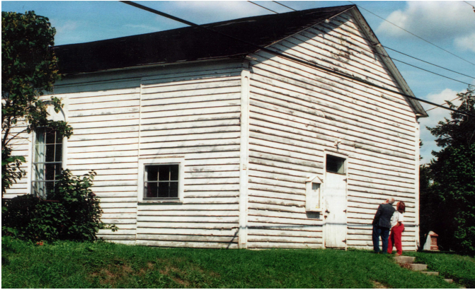
Photo: Diane Brisley Ted Davie and Diane Brisley assessing the condition of St. Paul's, then the Parish Hall for St. Alban's Church 1997
